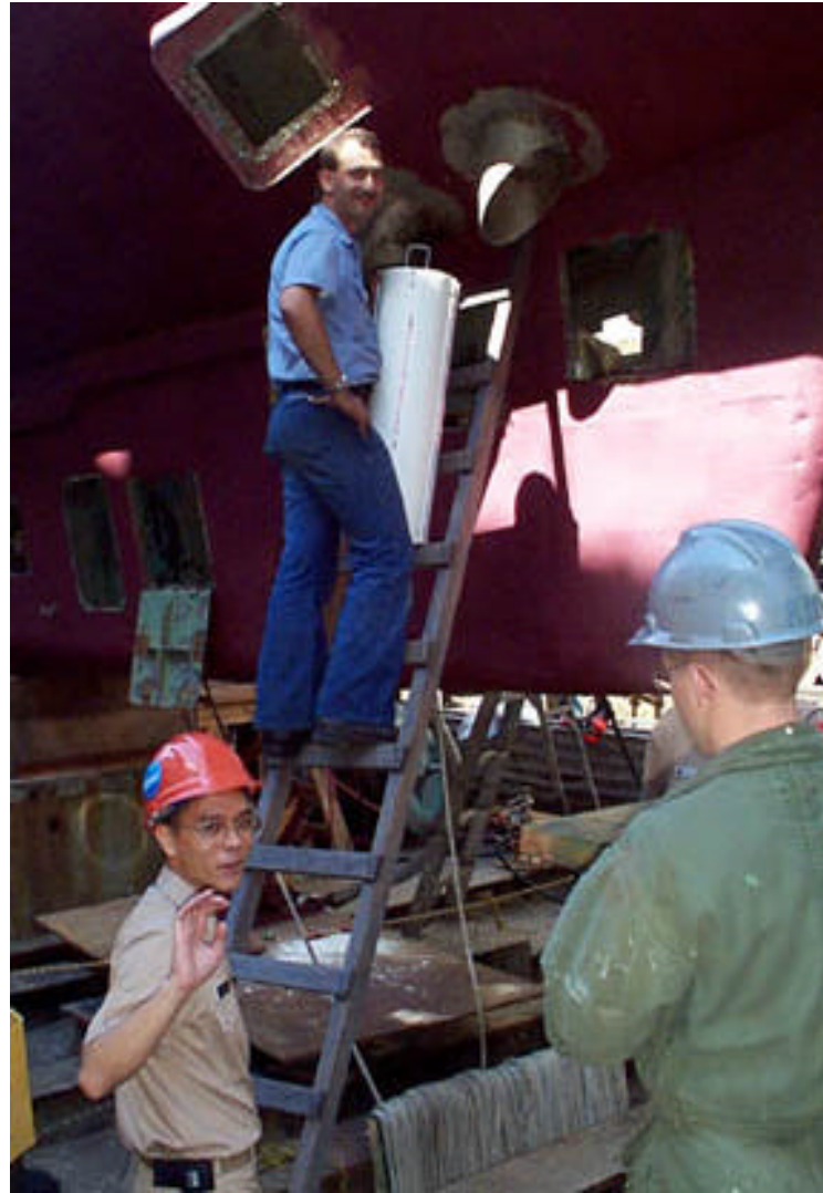
MIDN Evangelista and members of the NR-1 crew test fit UEC-1 to make sure that the mounting bracket and keyways are sized correctly.
